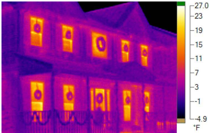
IR001025.IS2 12/18/2009 8:49:37 AM Windows – typical heat loss areas
