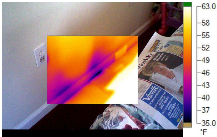
IR001041.IS2 12/18/2009 9:19:40 AM Air infiltration along baseboard
